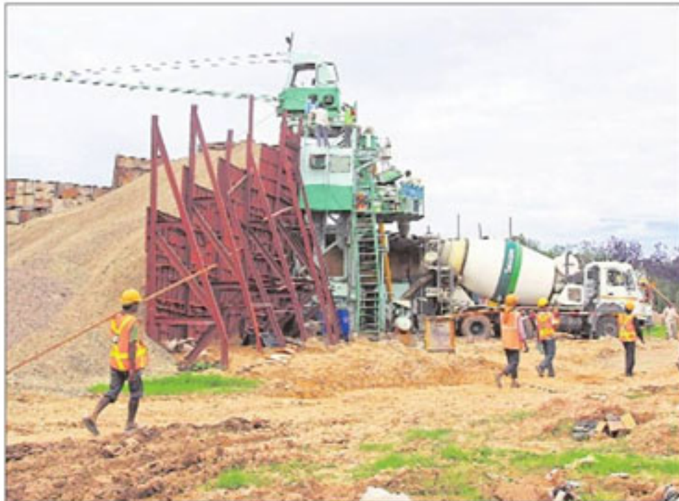
Construction on at the site of the Indian School of Business (ISB) Mohali campus at Knowledge City, Sector-81, Mohali.
